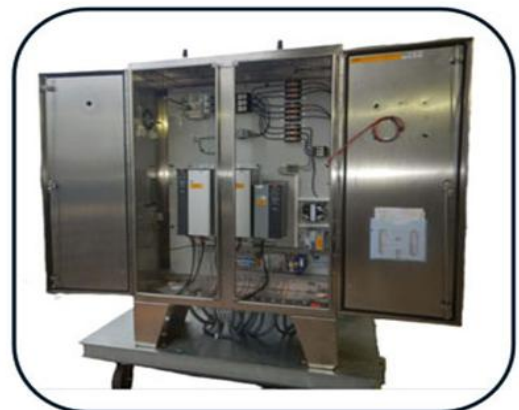
Control Panel Interior
